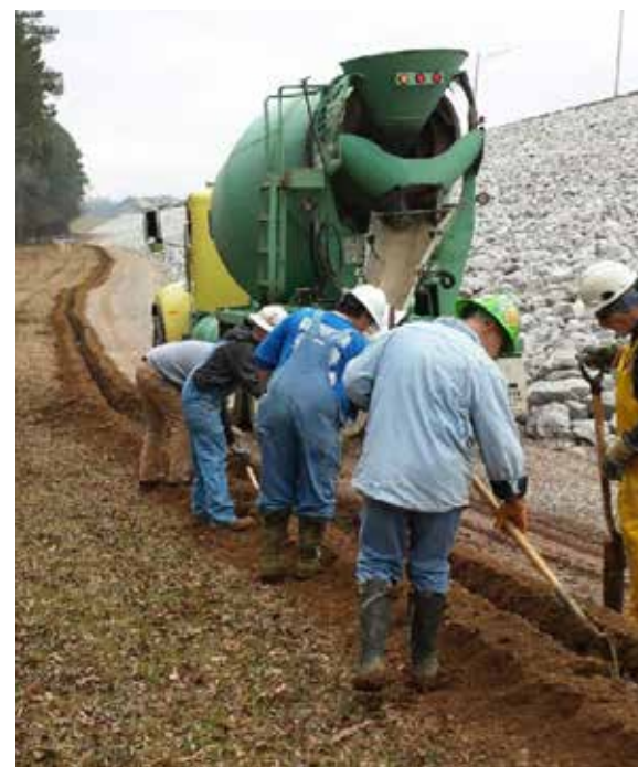
TVA crews install cables along Pickwick Dam's south embankment to detect even slight movement.
